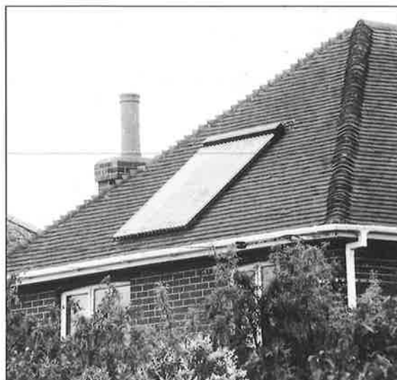
Solar panels on residential property
